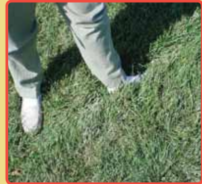
Figure 4.1. Holes in grassy area between a parking lot and hospital building
