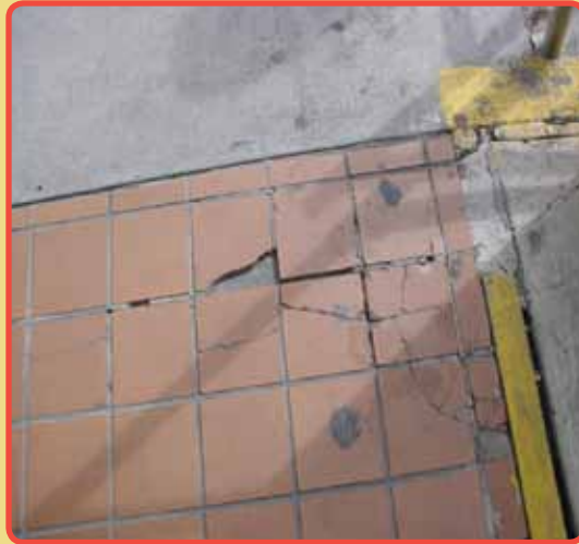
Figure 4.4. Cracked tiles in a walkway outside a hospital building
