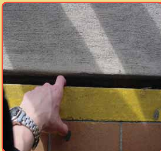
Figure 4.5. Large separation (greater than ½") in a walkway outside a hospital building
