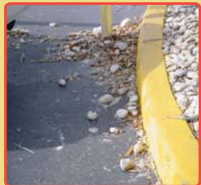
Figure 4.3. Stones and debris on walking surfaces in a parking lot
