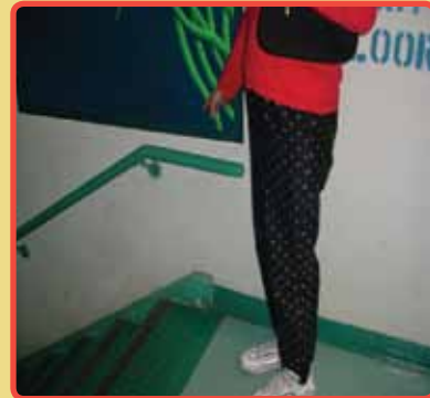
Figure 7.1. Handrail was lowered in order to hang large picture above; handrail too low to be of use
