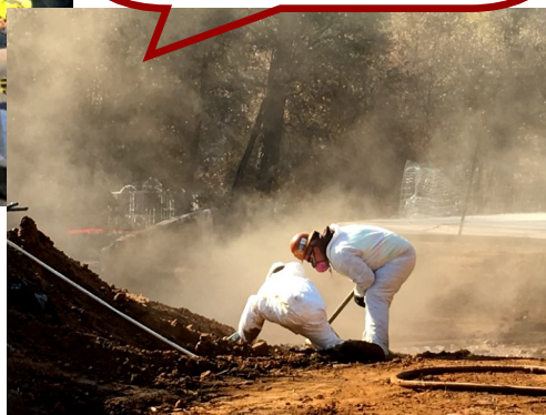
Two employees working inside the lot footprint with no dust suppression, surrounded by dust that may contain silica. Photo by NIOSH.
